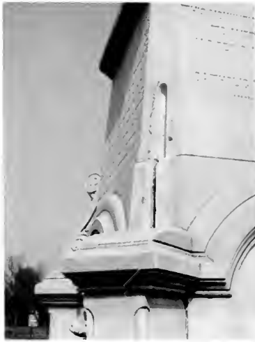
Figure 31: Missing scrolled bracket from pedestal (Photograph by author, March 2002)
